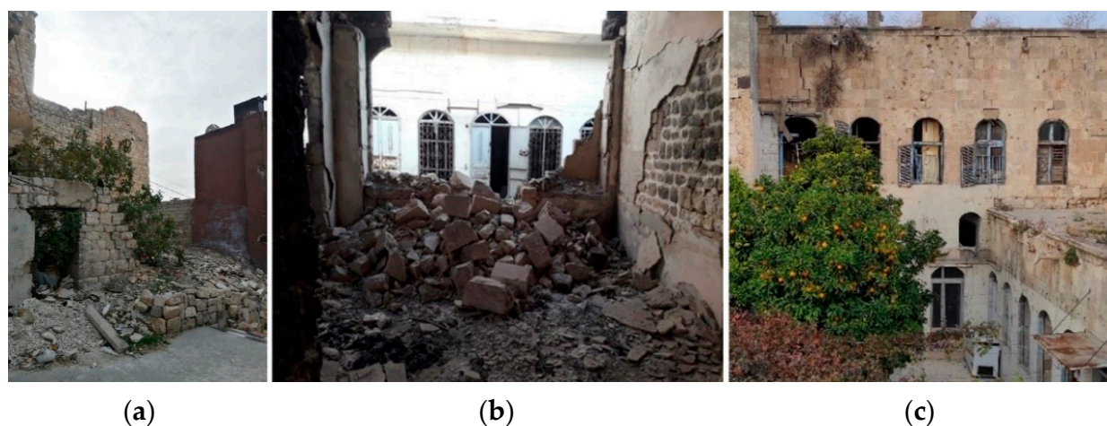
Figure 4. A house that was completely destroyed, Cadastral number 1426 (a); a house that was severely damaged, Cadastral number 1429 (b); bullet holes from the fighting, on the façade of the house at Cadastral number 1424 (c); Al-Aqaba neighborhood, Old Aleppo, Winter 2020, Source: C. Kousa and students' work.
