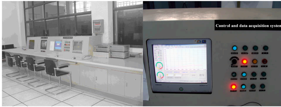
Fig. 5. Wind tunnel wind speed control system.
