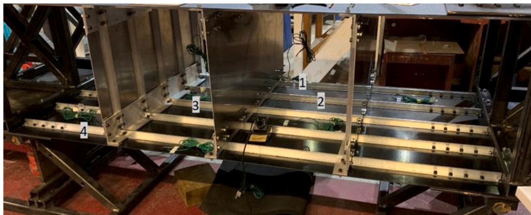
Fig. 13. Location of debonded stiffeners.
