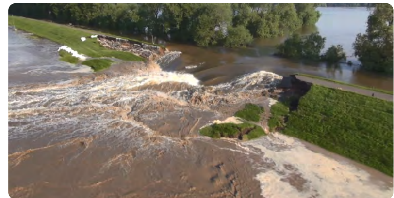
Figure 1: Dike failure in Breitenhagen, Germany. Photo by Weichel (2013) .
