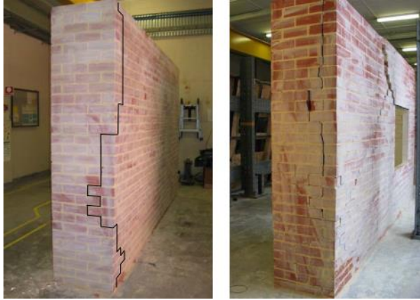
Figure 6.10. Examples of a mix of line and stepped cracks along the lateral edges of walls (Vaculik, 2012).
