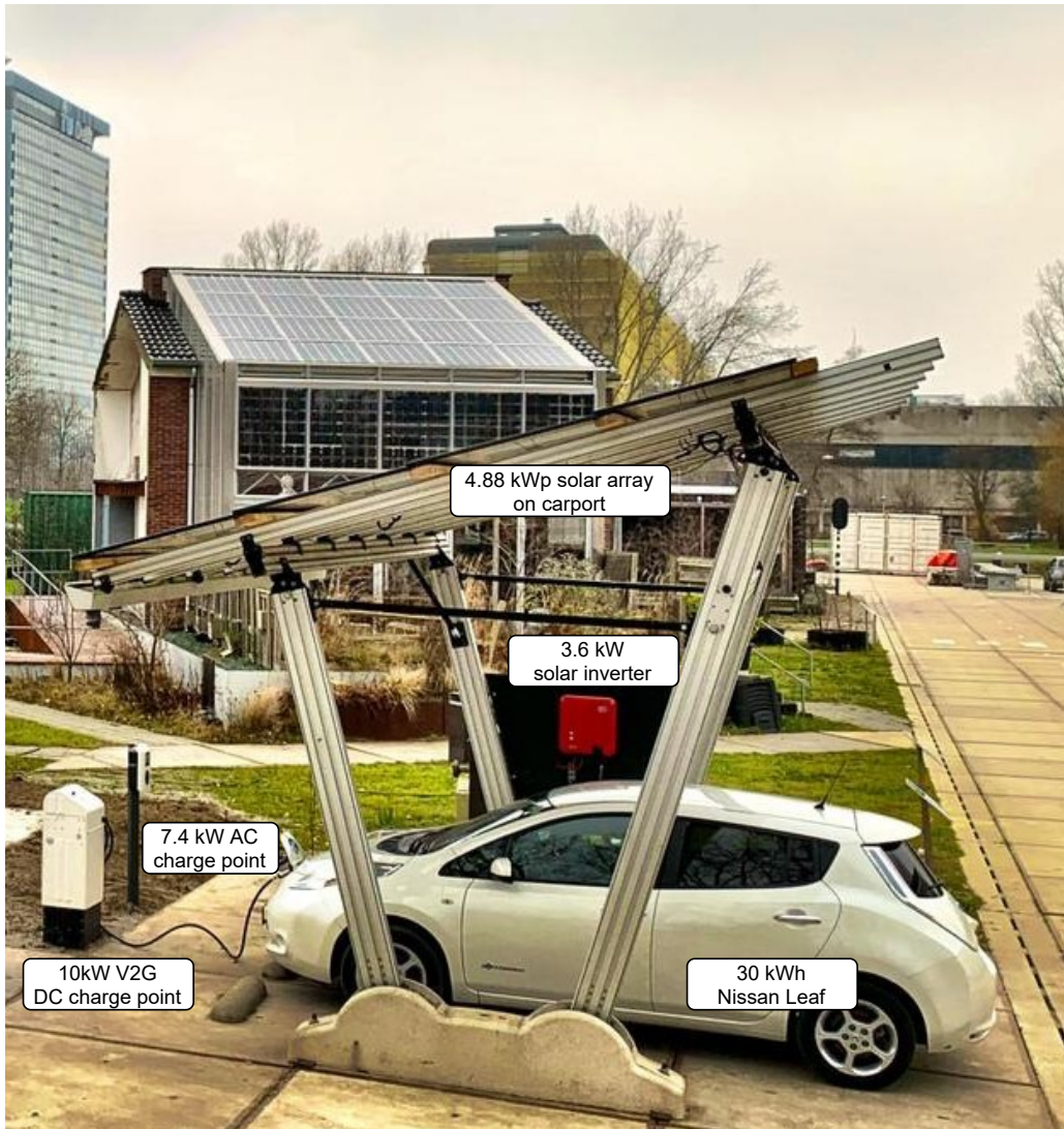
Figure 7.3: V2G test set-up at the solar carport located at the Green Village, TU Delft (Image courtesy of The Green Village)
