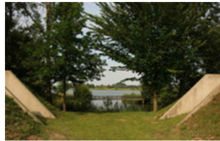
FIG. 4.93 Culemborg (NL), Werk aan het Spoen: openings in the earthwalls connecting with the surrounding waterline landscape (F. Marulo 2019)
