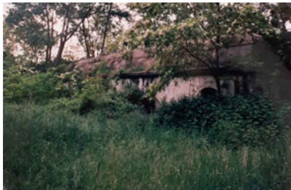
FIG. 5.19 Venice (IT), Forte Bazzera: the state of the fort after the abandonment of the military (1996) (ACCTM, Fond 1, Box Forti di Terra , File Forte Bazzera )
