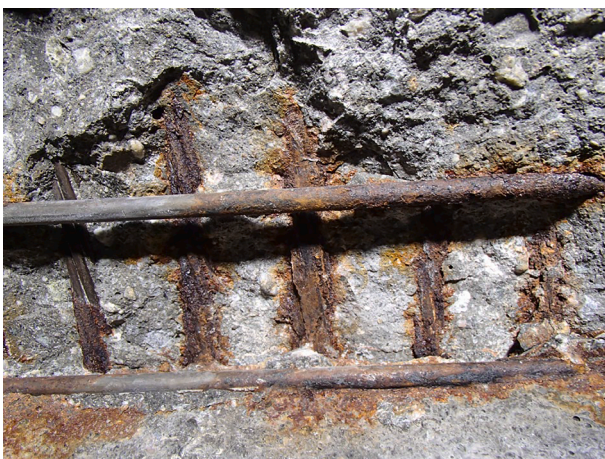
Fig. 7. Corrosion in the bottom layer of strands found near the middle support in an NIB girder in Hafrsfjord Bridge near Stavanger.
