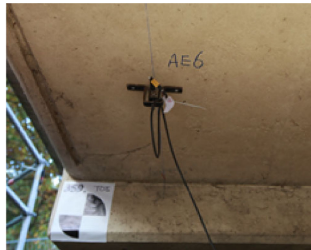
Figure 21. Installation of AE sensor in a proof load test in the Netherlands.
