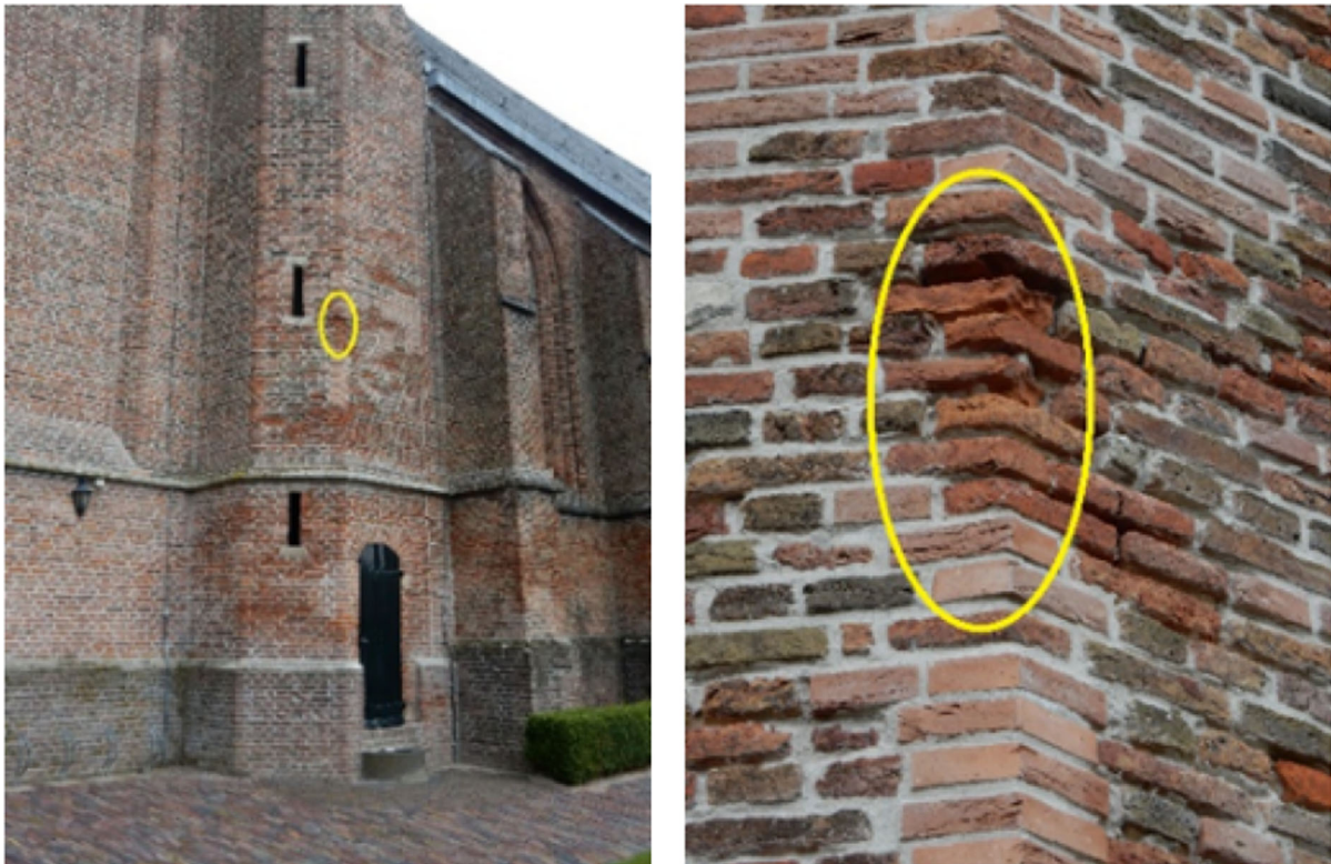
Fig. 21 Situation of the damage in 2016. Left, the reddish parts of the masonry indicate where the repointing is damaged. Right, detail of one of the spots with damaged repointing
