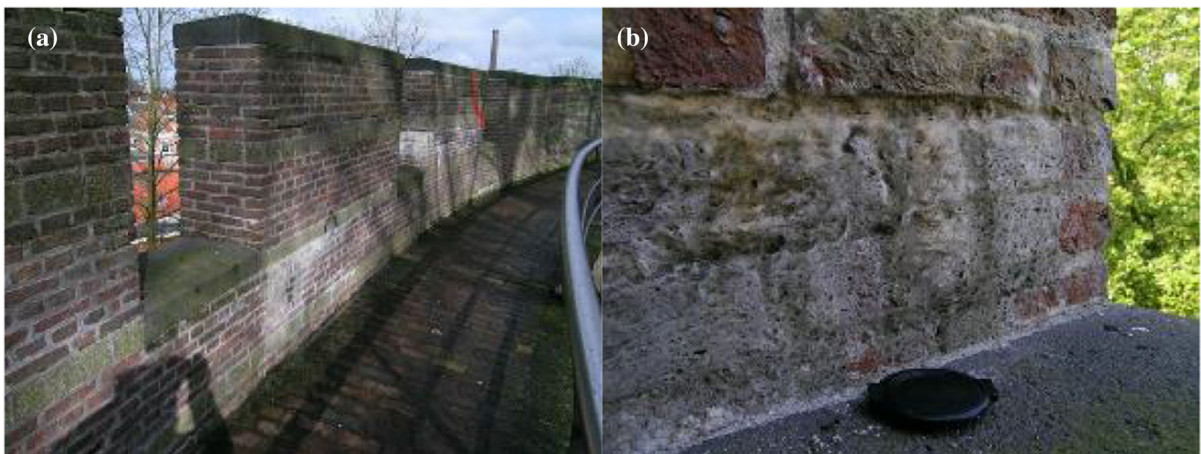
Fig. 32 a) Encrustation, due to leaching of mortar in very exposed masonry, the battlements of a motte castle; b) Detail
