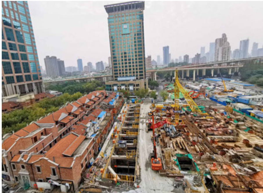
FIG. 6.30 Shangxianfang, one of the first listed Cultural Relic Protection Units (CRPU) for being a post-treaty residential neighbourhood, is under construction and transformation to become a luxury hotel. Source: author, 2021.
