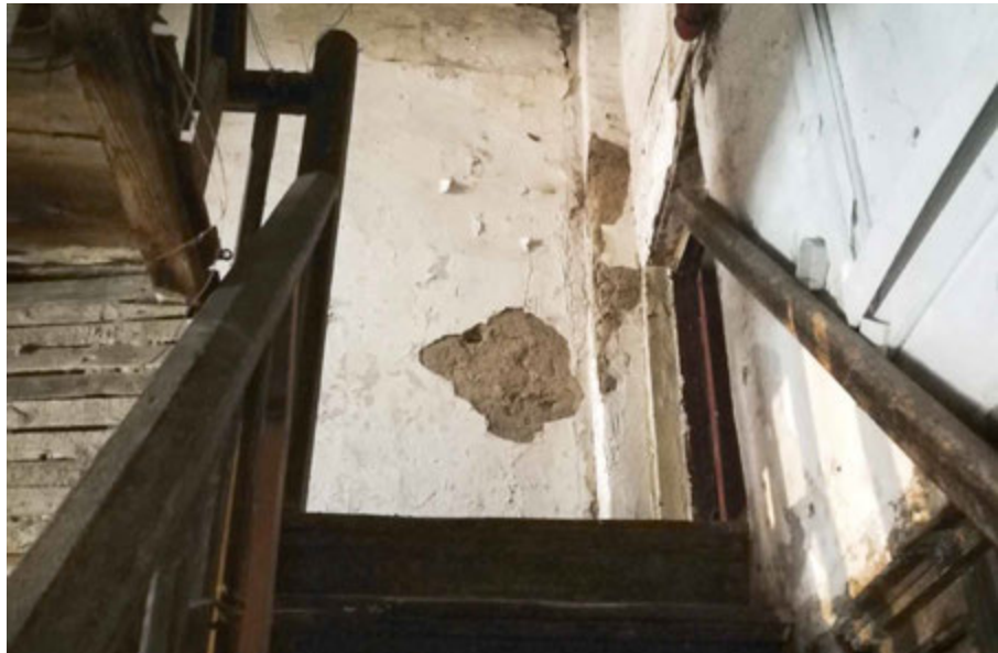
FIG. 8.19 The decayed staircase inside of a building in Bugaoli Source: author, 2018.
