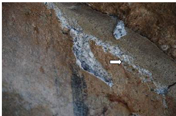
Fig. 5 Detachment of a lime-based plaster from an internal plaster layer. Archaeological site of Dion, Greece (Roman period): Plaster consisting of two layers of a total thickness of 2.5 cm (external: 0.5 cm, internal: 2 cm) with the external layer decorated with wall paintings (Photo archive: Lab of Building Materials AUTH)
