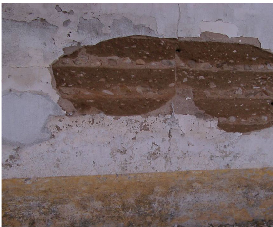
Fig. 2 Delaminated lime-based render with loss of plaster on earth-block masonry in Santarem Building, Portugal. Photo by A. Velosa
