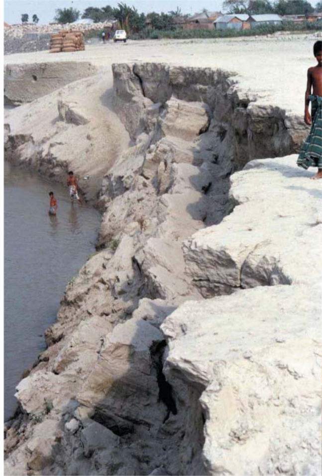
Figure 20.29 Large-scale slab failure by bank undercutting near Shailabari (~4 km upstream of Sirajganj). Photograph taken at low flow. During seasonal floods, the water level would be up to bankfull.
