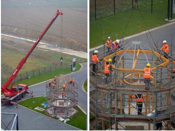
Figure 8 - 9. Building the outer framework of H4aC - A crane truck is lowering the dome for the main module. A similar dome is attached at the underside creating a symmetric volume. Photos: Steven Vandenbulcke
