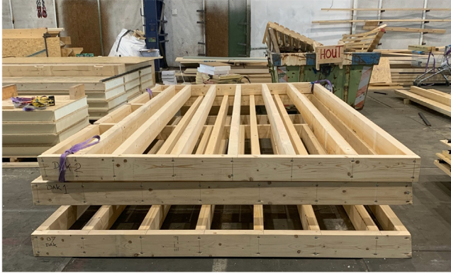
Figure 10.6 Timber frames, stacked in the factory, before the insulation and sheathing boards are applied.
