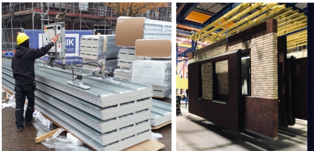
Figure 10.4 (A) Prefabricated roof panels used in the construction of the 12 zero-energy dwellings, in Vlaardingen, the Netherlands. (B) Completerc RC Panels ( Rc Panels, 2021 ) with weather finishing of brick tiles.
