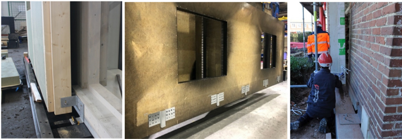
Figure 10.3 (A) The panels are connected to wooden posts, attached to the existing structure with steel U profiles. (B) Anchors on the back of the façade panel, to be connected on rails attaching to the existing building. (C) The installation of the prefabricated panel on the concrete block that bears the extra weight. Hem, France, Net-zero retrofit, under construction, Vilogia.
