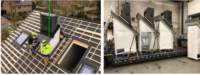
Figure 10.11 Preassembled building services unit placement on the roof. Factory Zero, the Netherlands, energy modules.
