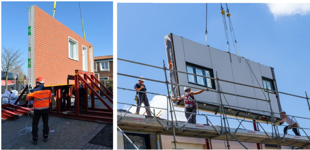
Figure 10.7 (A) The installation of the prefabricated panel on the existing façade. Hem, France, Net zero retrofit, under construction, Vilogia (B) Longueau—Rénovation thermique E = 0.
