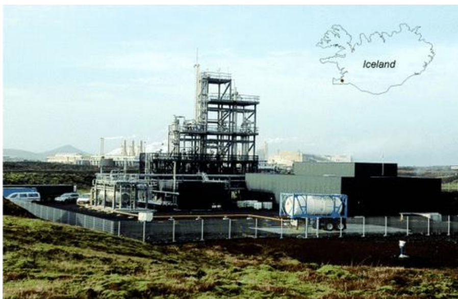
Figure 1.2 The “George Olah Carbon Dioxide to Renewable Methanol Plant” of Carbon Recycling International in Iceland based on local geothermal energy. The first commercial carbon dioxide recycling plant operating in the world. 7
