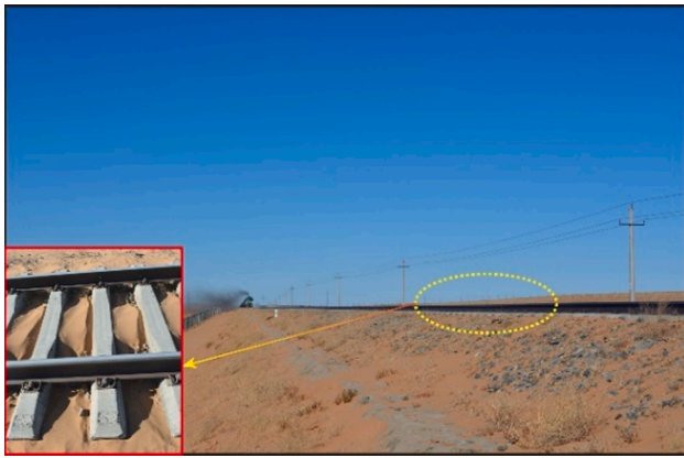
Fig. 1. Windblown sand railway line in Northwest China.
