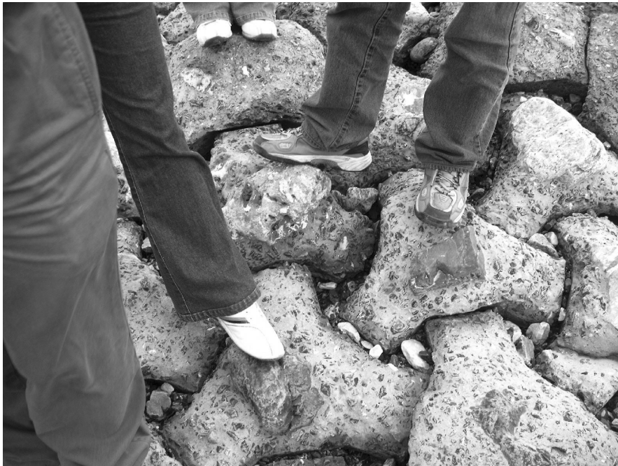
Figure 8-28 The same blocks as in Figure 8-22, but after three years in service
