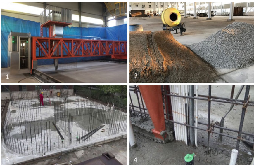
Fig. 2.23 On-site 3D-printing by HuaShang Tengda: 1. gantry-based printer with a hopper on the top of the printhead; 2. raw materials and mixer; 3. foundation and connective steel bars; 4. deposition of the first layer
