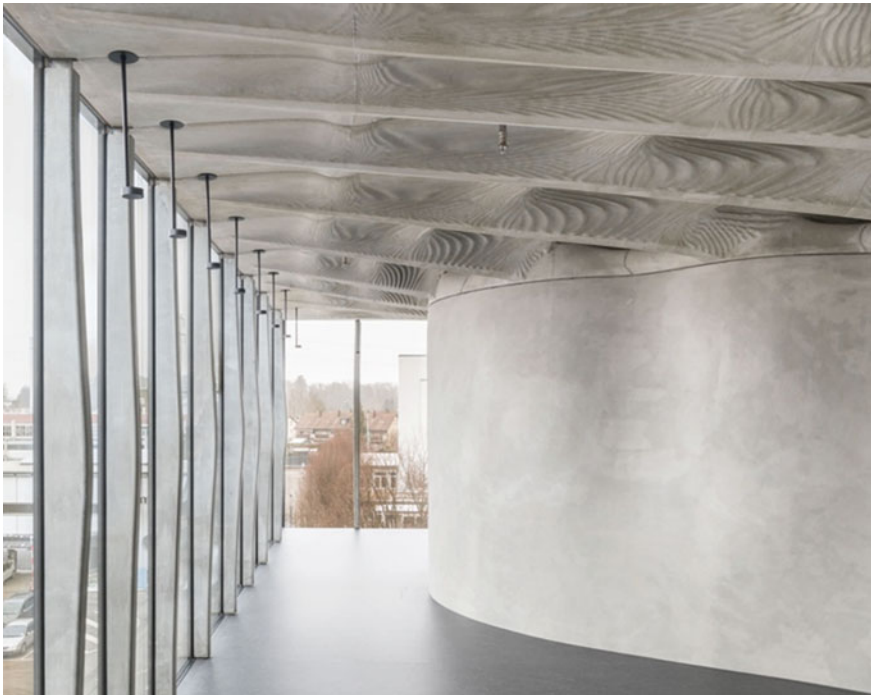
Fig. 2.16 Final installation of façade mullions in the DFAB House, on the left-hand side of the image
