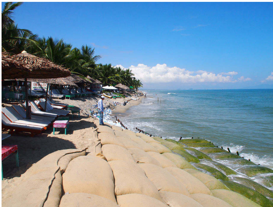
Figure 10.21: Cross-shore and longshore damage to an incorrectly applied revetment, Cua Dai beach, Hoi An, Vietnam, around 2016. Photo by Marcel J.F. Stive ( Credits on page 575).
