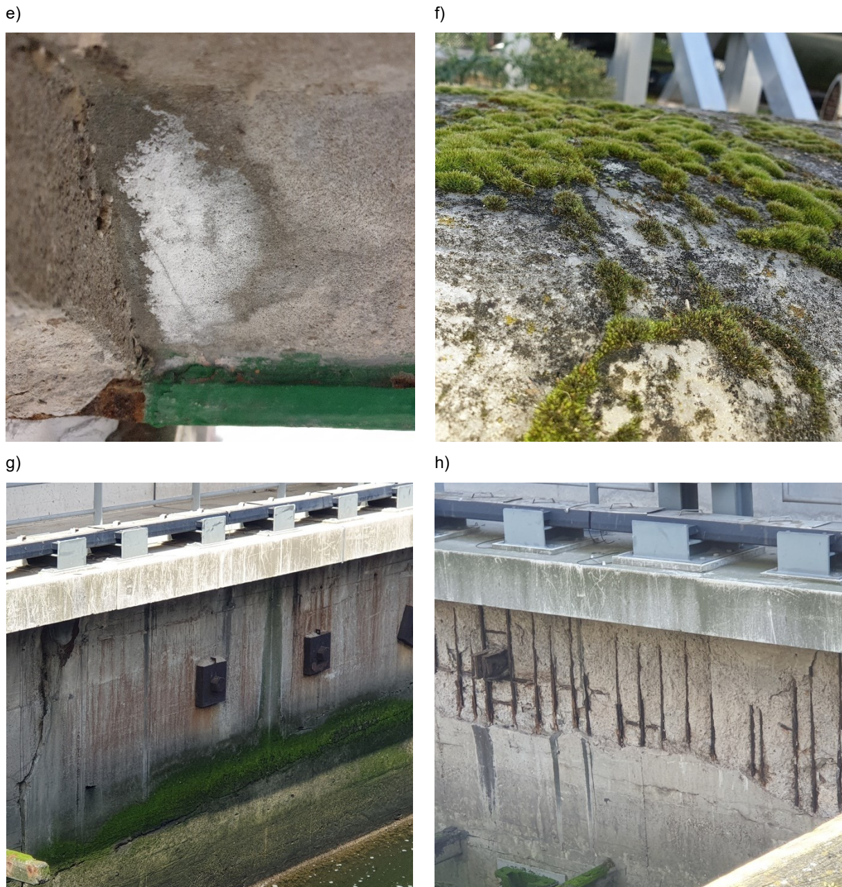
Fig. 8. Concrete surface texture examples: (a) newly built reinforced concrete and formwork marks, (b) spall, (c) white paint, (d) remained coating, (e) efflorescence, (f) algae, (g) crack, dirt and rust stain, (h) steel corrosion and concrete cover damage
