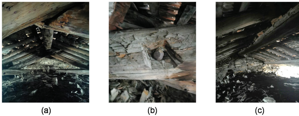
Figure 4. (a) Existing wooden roof structure; (b) existing metal pin between timber struts and ties; (c) ridge beam undergoing excessive deflection.
