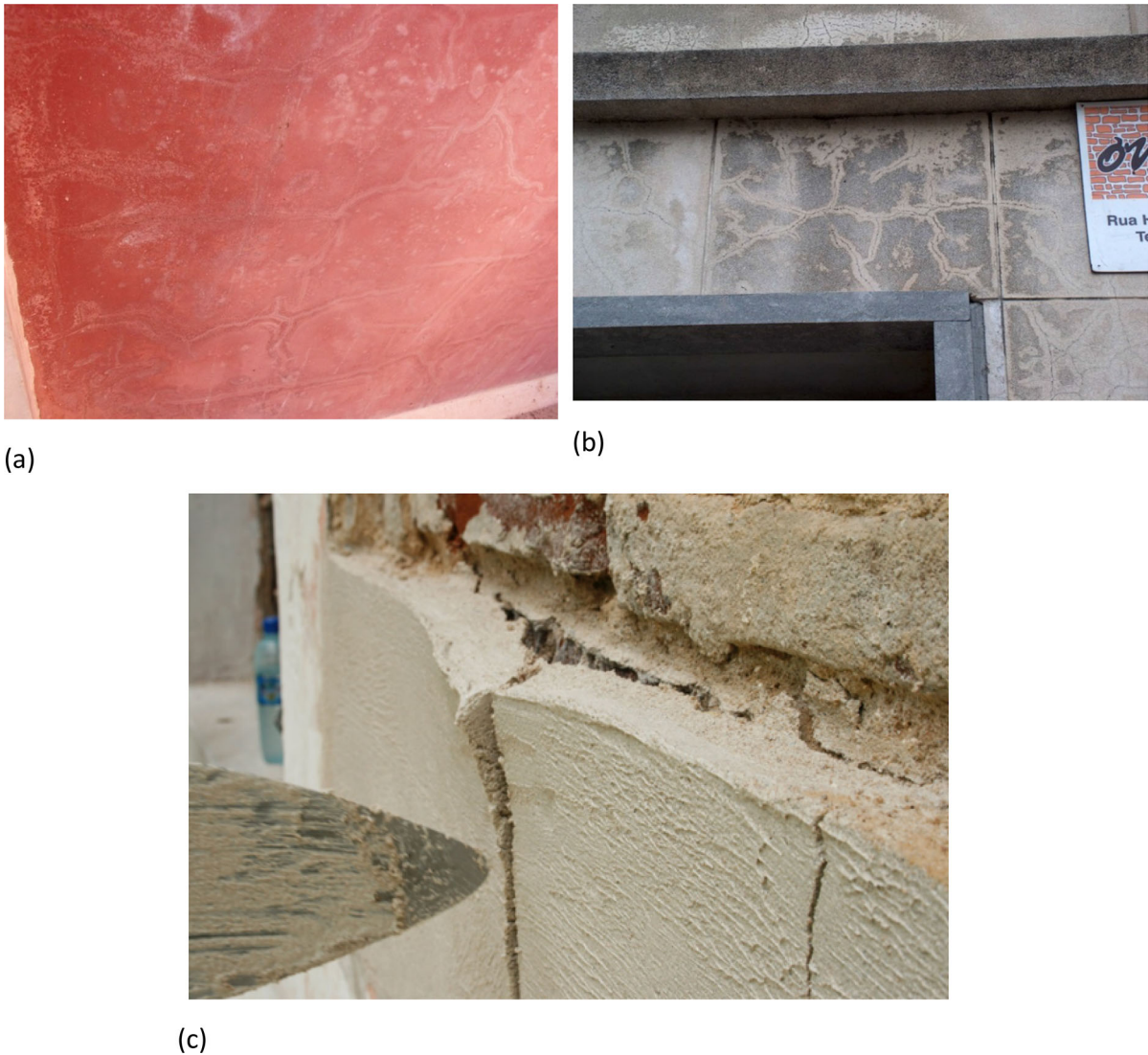
Fig. 10 Different examples of cracking problems due to restrained shrinkage in lime-based renders. (a) cracking of a thin finishing coat producing fine cracks on the thin coat very visible due to the finishing colour; (b) cracking of the render
