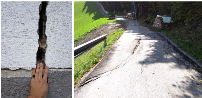
Figure 1.4: Damage to a house (left) and infrastructure (right) in Vögelsberg due to slope movement. (left: image courtesy of Thomas Zieher, right: image by the author, October 2018)
