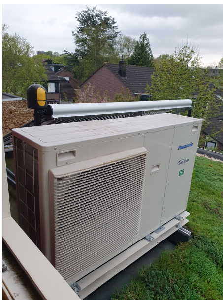
Figure 6.2: View from roof of retrofitted house. From left to right: solar boiler, heat pump and sedum roof cover (picture by first author).
