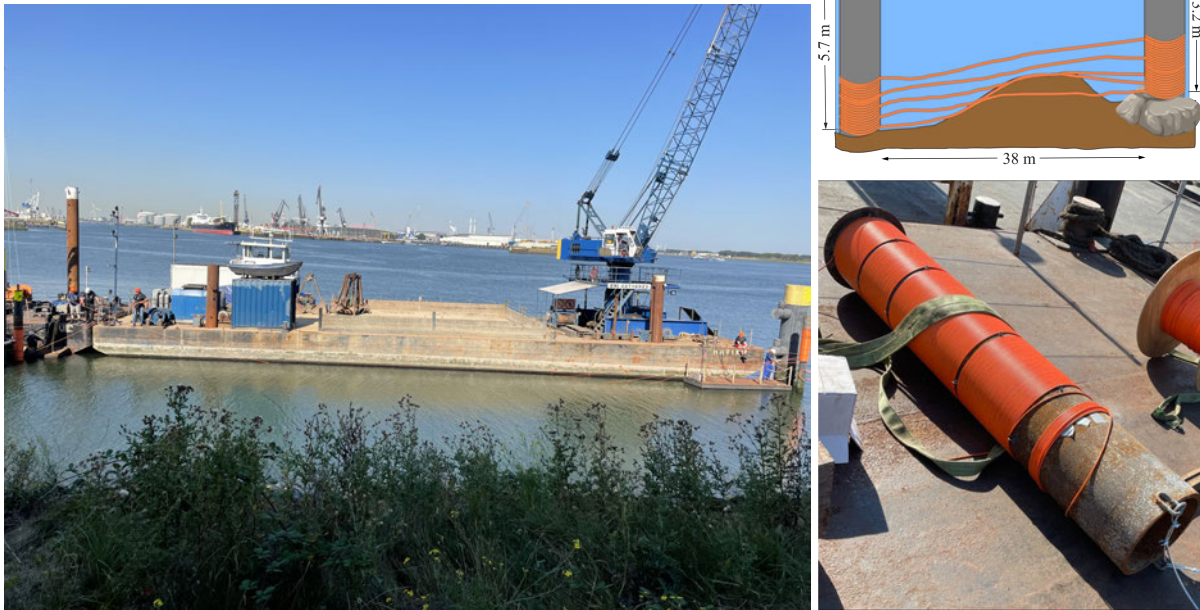
Figure 1 Left: two mantels with the direct burial single mode fibre being lowered onto the steel poles. Top and bottom right: sketch of the setup and a picture of a mantel with the fibre.
