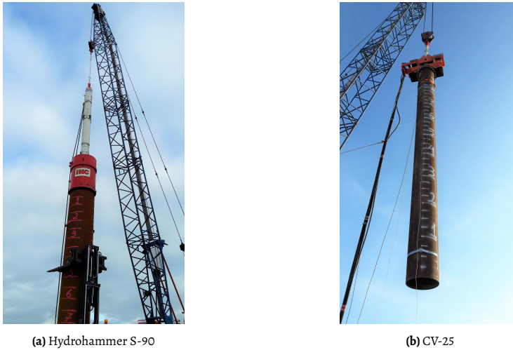
Figure 1.2: (a) Impact hammer and (b) axial vibratory device mounted on the top of tubular piles from the GDP field campaign.
