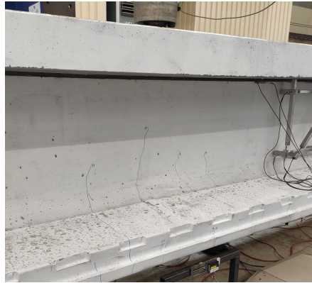
Fig. 4. Damage level 1. Crack pattern
