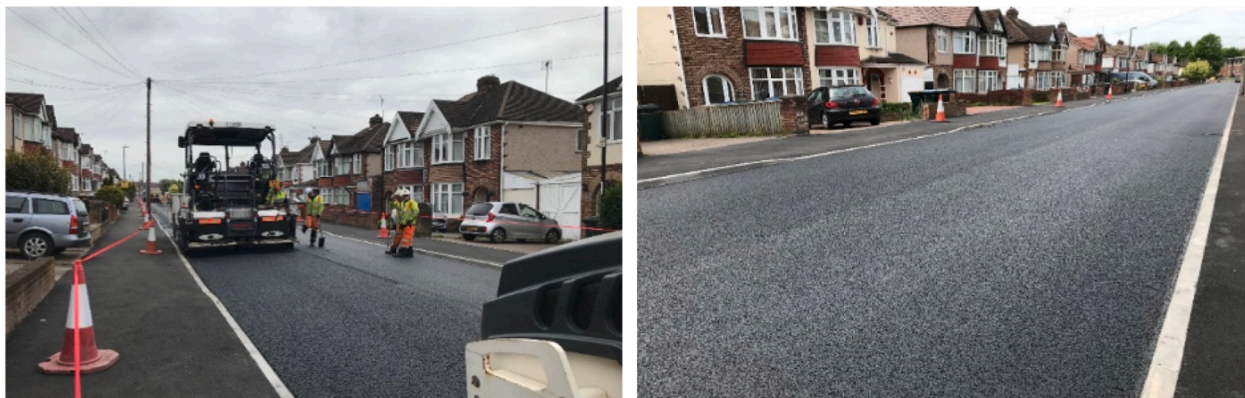
Fig. 6. Trial section with asphalt mixture containing waste plastic in Coventry City Council, UK [143].
