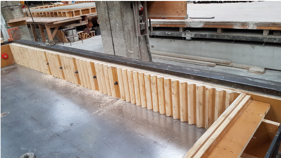
Figure 3.5: Wooden ribbings in the edge side formwork for the Aligned small shear key connection of a precast concrete large panel element
