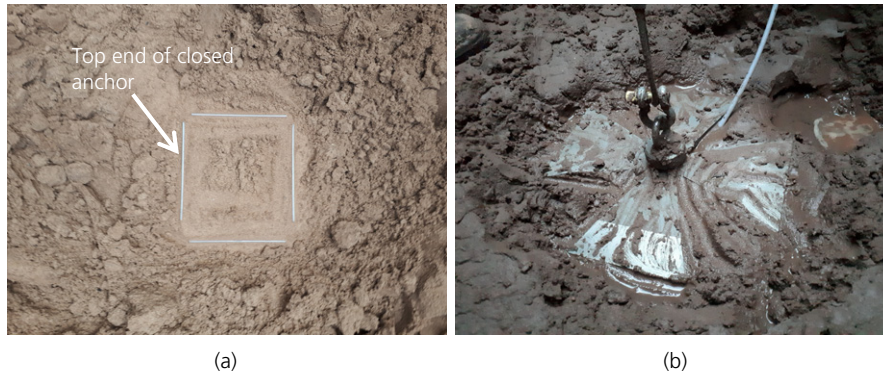
Figure 9. Photographs of the unearthed anchor: (a) closed after installation; (b) fully opened after pull-out
