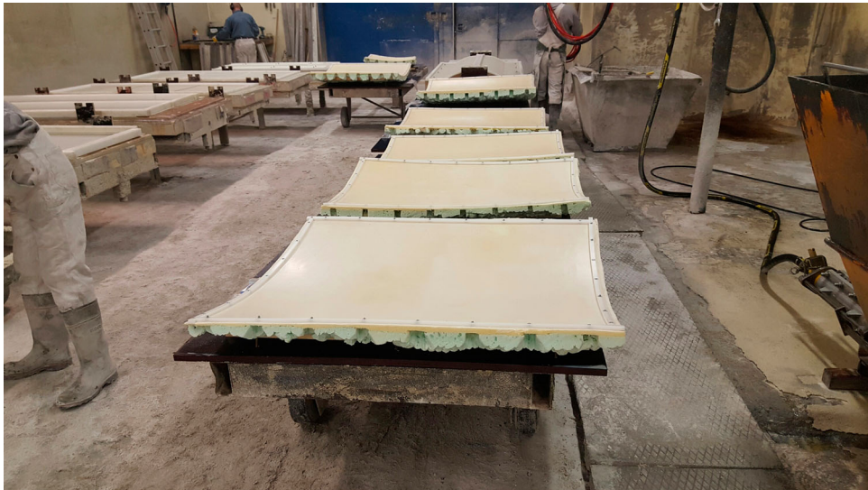
Figure 35. Intermediate mould for ring 3–9 of the thin-walled GFRC hyperbolic shell before the first casting.
