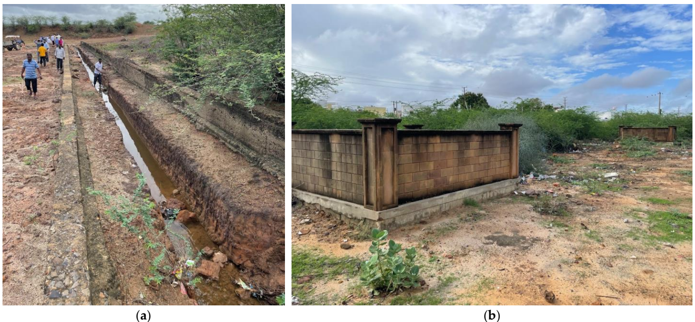
Figure 3. (a) A 500 m long drain discharges water from Umasar Lake toward the qanat system of 24 wells, of which two are depicted in image (b), to transport the water underneath a hill toward Hamirsar (authors 2022).
