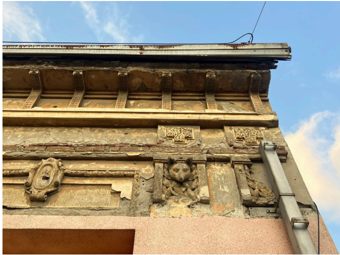
Fig. 1. Ornamental details of houses that are falling slowly apart, 'rotting quietly and unnoticed' in downtown Osijek. Photo: Angeliki Sioli, August 2022.
