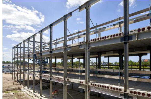
Figure 4: Use of donor skeleton on a large scale for Biopartner in Oegstgeest (The Netherlands) (source Imd/ Rene de Wit)
