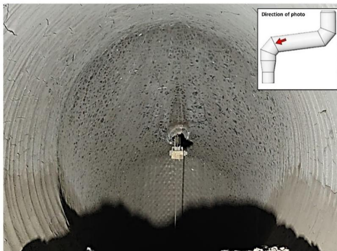
Figure 5-9. Wall condition around the oxygen lance and first bend of the dog-leg geometry (inspection 2019)
