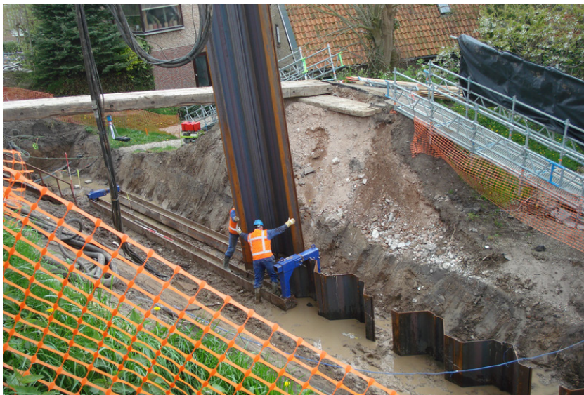
Figure 18: Installation of sheet pile walls at the inner toe of an embankment near Ammerstol, the Netherlands.
