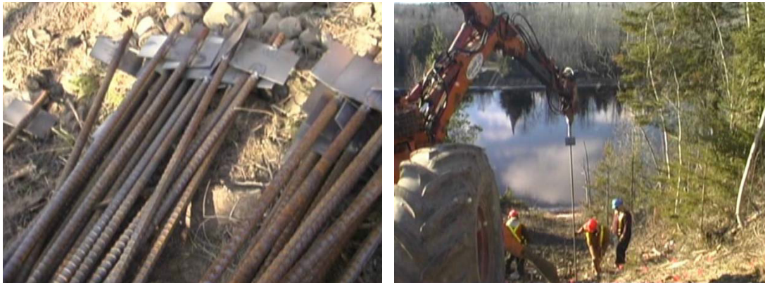
Figure 19: Left: Soil nails of 35 mm with a plate for extra resistance against shallow soil flow. These were used to stabilize a 30 m high riverbank along the Kaministiquia river in Canada, with nails in a grid of 1 m to 1.5 m. Right: nails were installed using percussive hammering (Fabius et al., 2008).
