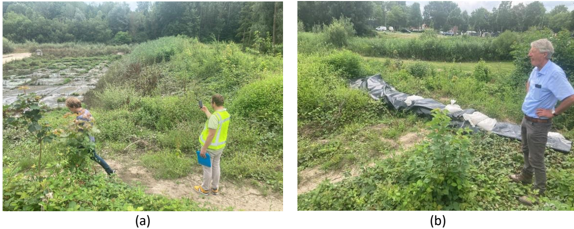
Figure 12 De Dem water storage basin with (a) the outflow location in the bottom right-hand corner of the photograph and (b) traces of erosion in the same location (photographs provided by Bas Jonkman, TU Delft).
