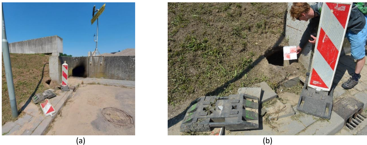
Figure 7: Signs of internal erosion at the junction between two different retaining walls: (a) overview showing the lower and higher retaining walls, (b) detail showing the hole left behind (the red and white blocks on the card each measure 10 by 10 cm).
