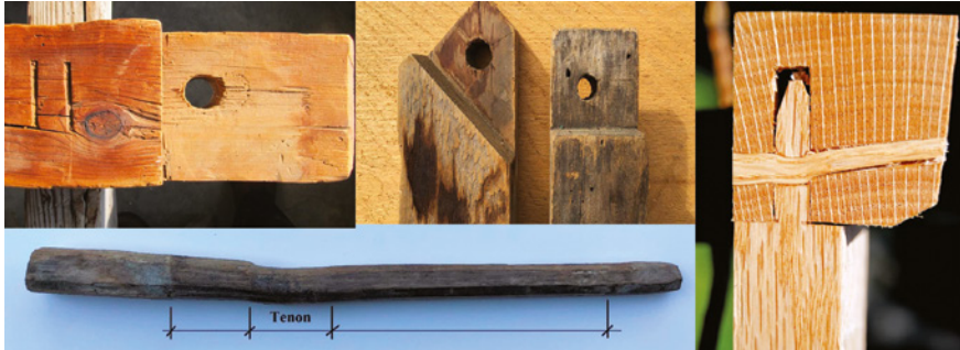
FIGURE 6 Examples of drawbored joints. (Top right) The peg holes location is pricked onto the tenon on a Dutch barn frame from 1801 made out of eastern white pine; (top middle) Clearly visible layout markings on these two tenons, left in red Red Spruce from around 1855, right in a Sugar Maple rafter from around 1820 (top right) Cut through a drawbored joint in oak, clearly visible deformation of pin drawing the mortise into the tenon (Lost Art Press 2021); all others (Sobon & DeStefano 2020)
