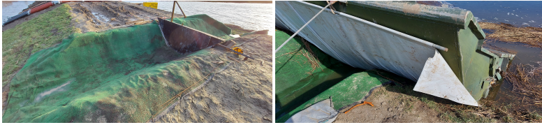
Figure 3.7: (left) Weir to regulate water through breach, (right) BresDefender with white tarpaulin
