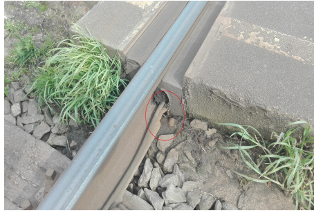
Figure 3.2: Reduced profiles in rail foot caused by corrosion [2].
