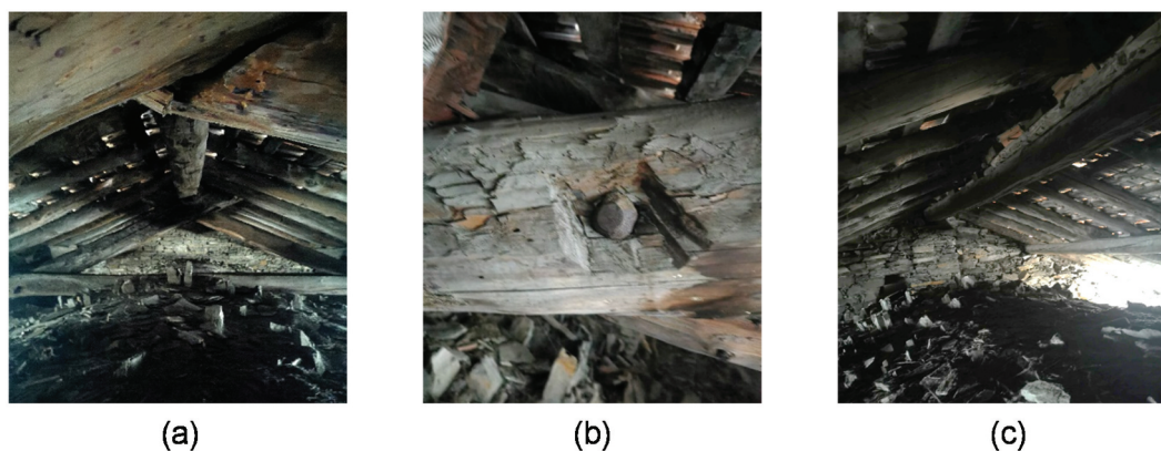
Figure 4. (a) Existing wooden roof structure; (b) existing metal pin between timber struts and ties; (c) ridge beam undergoing excessive deflection.
