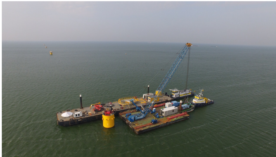
Figure 8: Aerial photo showing the shaker on pile W27, the mobilized barges and crane.
