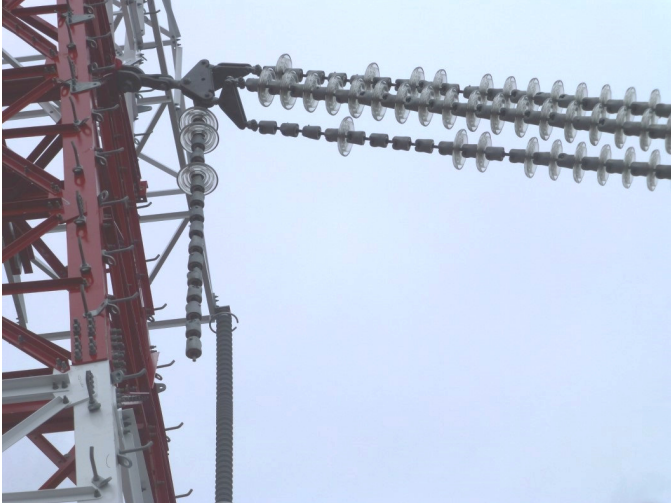
FIGURE 3 - Insulator string failure on Storfjord crossing
