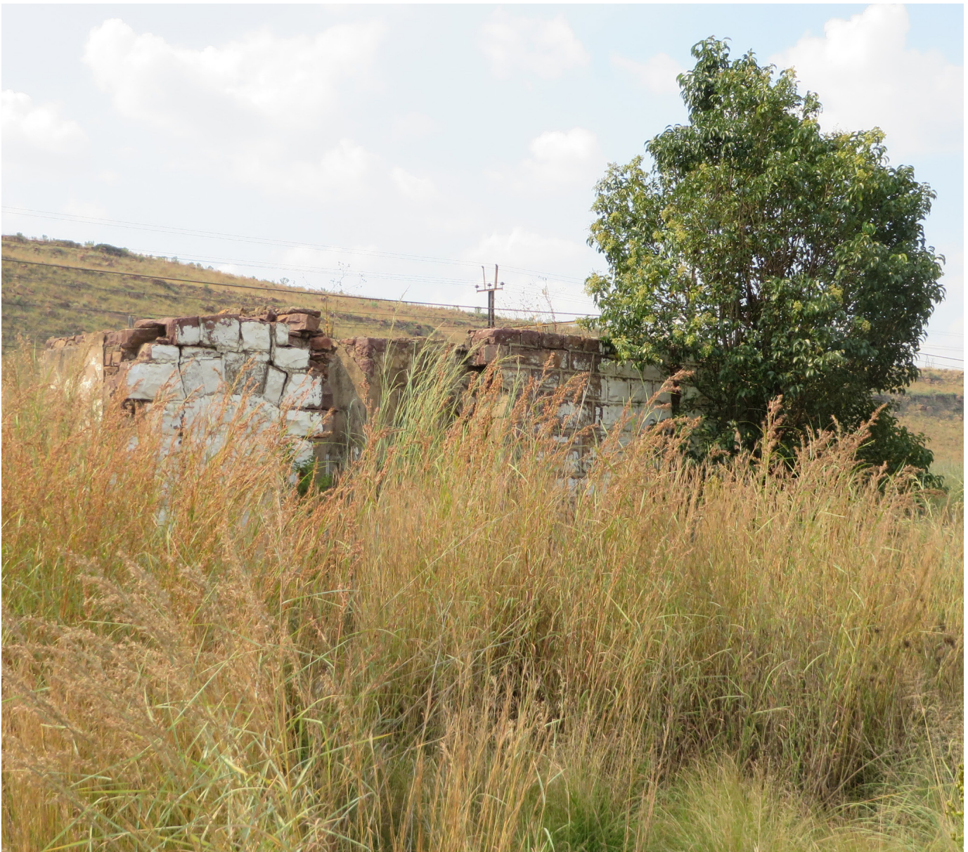
03.04 and 03.05: The double Gangers Cottage at Groot Olifantsrivier Station (NZASM_EL_135) has all but totally disappeared in the thirty years between 1986 and 2016. (3.04 De Jong, RC)
