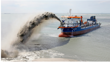
Figure 1.1: Vox Maxima, owned by dredging company Van Oord, constructing an island using the method rain-bowling.
