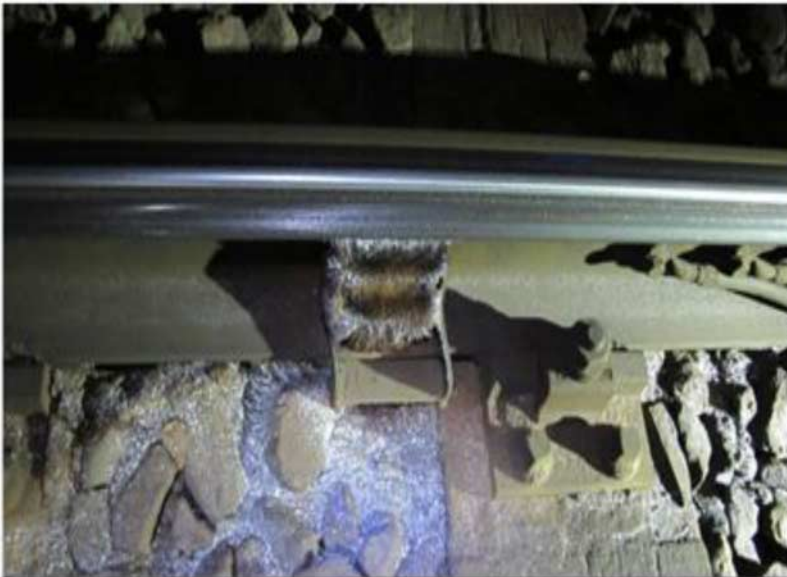
Figure 2. Severely worn narrow radius track section with wear debris at ballast and collecting magnet.
