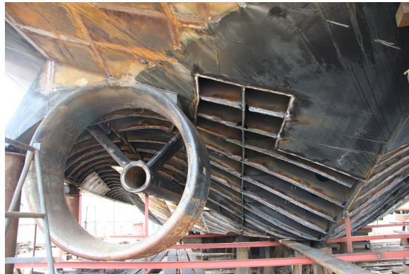
Figure 3.5: The tunnel of an double propeller inland ship under construction. The tunnel frames can be identified and by taking the highest point in each frame, one can draw the tunnel top curve and see that for this specific ship, the tunnel is such that the flow enters the duct and propeller under an angle. (photo by René Rapati, Groenendijk & Soetermeer)
