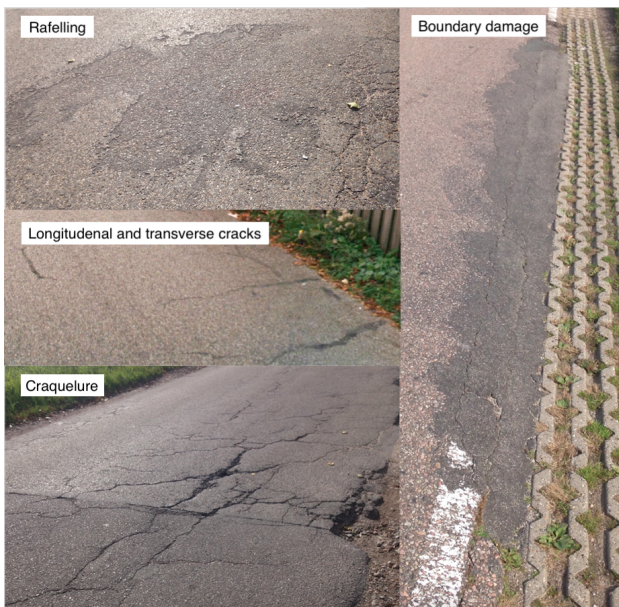
Figure 1. Examples of road surface damage.
