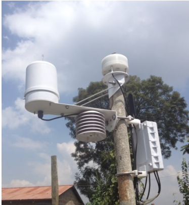
Figure 10: TAHMO installed at a Kenyan farm
